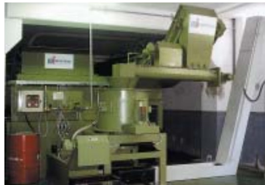
Central filter processing plant pumped by MRS pump back stations
